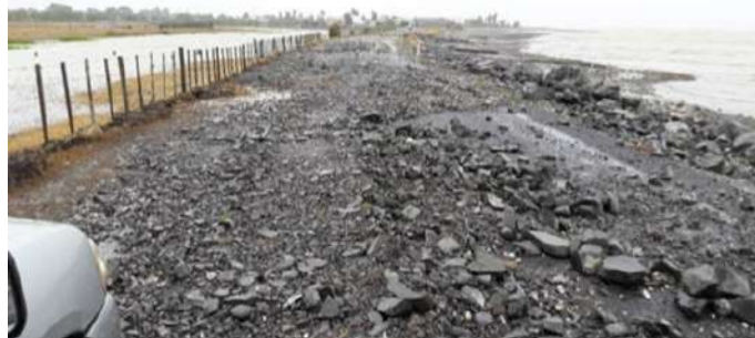
Damage to East Coast Road, Anarau Bay.
